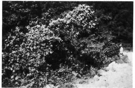
Photo. 4 Experimental plot No.2 on banking slope of forest road construction in 1971 (Oct. 6, 1985)
